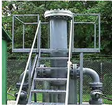
Coalescing filter in service cleaning an eight inch gas pipeline in the midwestern US.
